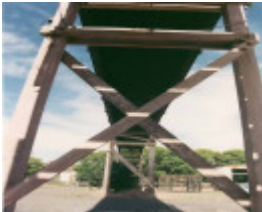
B7125 Nth Fitzroy Railway Footbridge
