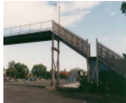
B7125 Nth Fitzroy Railway Footbridge
