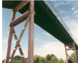
B7125 Nth Fitzroy Railway Footbridge
