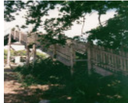
B7125 Nth Fitzroy Railway Footbridge
