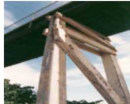
B7125 Nth Fitzroy Railway Footbridge
