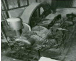
B6329 Rokeby Pumping Station
