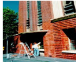
former royal australian army medical corps training depot a'beckett street melb facade detail
