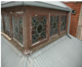
Before Photograph - Reference F3907 2014
