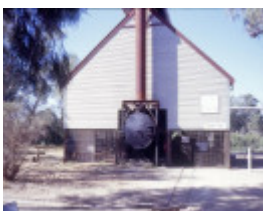
h00548 psyche bend pumping station psyche bend mildura smoke box and chimney base she project 2003
