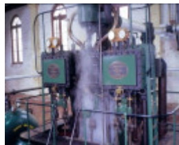
h00548 psyche bend pumping station psyche bend mildura engine room close up she project 2003
