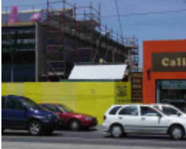
burnley bridge road burnley bridge road 514
