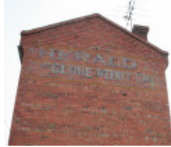
Fading Signage - 1 Groom Street.JPG
