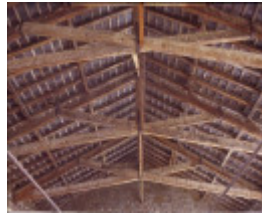
h00389 portarlington mill turner crt portarlington scissor beam construction under roof she project 2003
