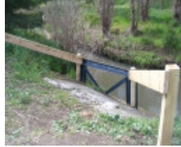
Remainder of bridge left on Alphington side of creek
