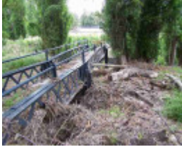
Former Darebin Creek Footbridge (immediately after 2006 flood)
