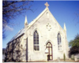
h00523 former methodist church ford st beechworth view from north she project 2003
