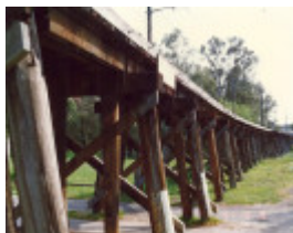
Railway Timber Trestle Bridge, Panther Place Colour - Shire of Eltham Heritage Study 1992
