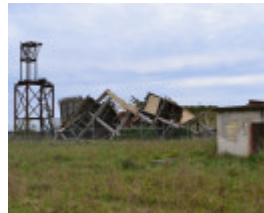
Wonthaggi Kirrak Area- Collapse Sept 2012
