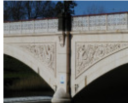
h01440 morell bridge anderson st over yarra river south yarra close up she project 2004
