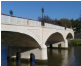
h01440 morell bridge anderson st over yarra river south yarra distant view she project 2004
