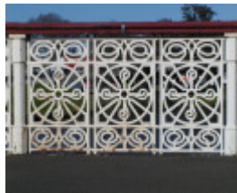
h01440 morell bridge anderson st over yarra river south yarra iron work she project 2004
