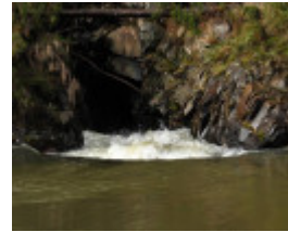
Inlet pool, rock bar and inlet of the diversion tunnel (north end of site)
