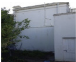
Before Photograph - Reference F3856 2014
