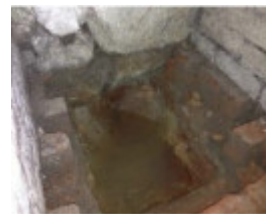
Before Photograph - Reference F3856 2014
