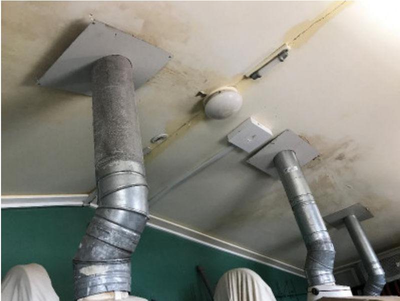
Memorial Hall Koroit, projector chimneys.JPG
