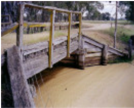
TU 01 - Timber Bridge, old Tulkara Navarre Road over Heifer Station Creek tributary, TULKARA
