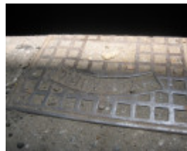
H2117 Overhead Water Tank Spencer St Power Station Hydraulic Valve Cover Plate 6 Dec 2006 mz
