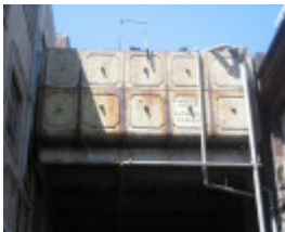
H2117 Overhead Water Tank Spencer St Power Station Front View Detail 6 Dec 2006 mz
