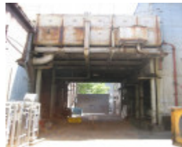
H2117 Overhead Water Tank Spencer St Power Station Rear View 6 Dec 2006 mz
