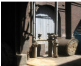
H2117 Overhead Water Tank Spencer St Power Station Associated Pipework 6 Dec 2006 mz
