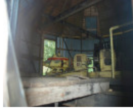
BAIRNSDALE PUMPING STATION SOHE 2008
