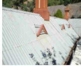
Before Photograph - Reference F3834 2014
