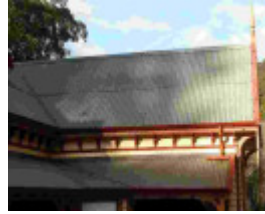
Before Photograph - Reference F3834 2014
