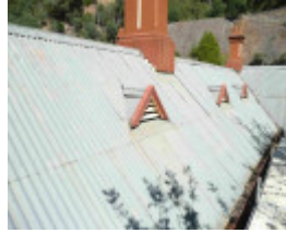
Before Photograph - Reference F3834 2014
