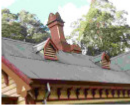
Before Photograph - Reference F3834 2014
