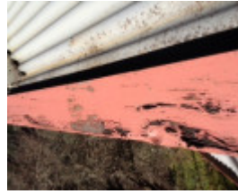
Before Photograph - Reference F3834 2014
