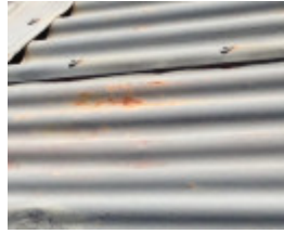
Before Photograph - Reference F3834 2014
