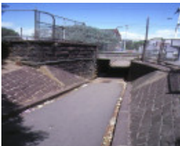
former albert park railway station complex ferrars street albert park underpass nov1986
