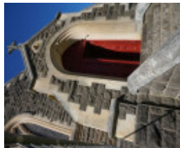
2023, Narthex, paint to door not original.
