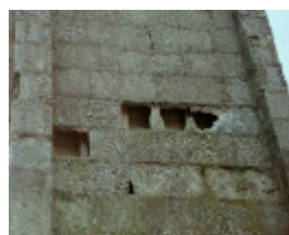
Snake Valley Wesleyan Tower Deterioration
