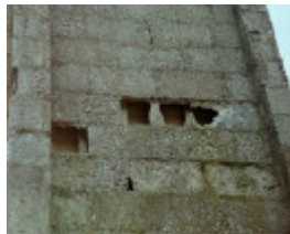
Snake Valley Wesleyan Tower Deterioration
