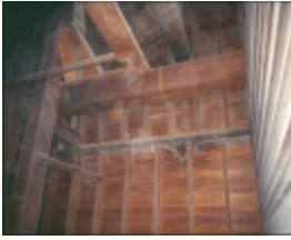
h02050 richmond maltings storage rooms and machinery mz june03
