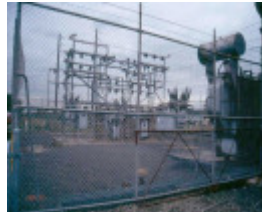
h02025 5 bunyip sub stationjul03 jc
