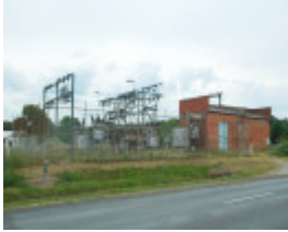
BUNYIP RAILWAY SUB STATION SOHE 2008
