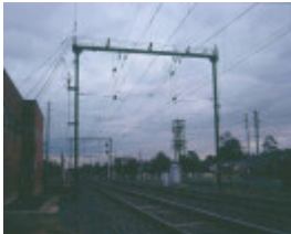
h02025 6 bunyip sub stationjul03 jc
