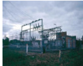
h02025 4 bunyip sub stationjul03 jc1
