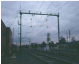
h02025 6 bunyip sub stationjul03 jc
