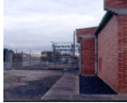
h02025 2 bunyip sub stationjul03 jc
