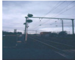
h02025 7 bunyip sub stationjul03 jc
