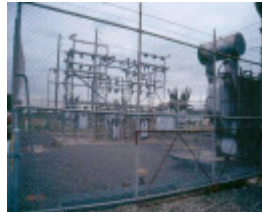
h02025 5 bunyip sub stationjul03 jc
