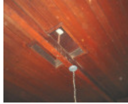
h01033 east view heidleberg ceiling vent nov2004 mz
