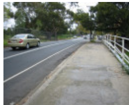
h02080 st kilda street bridge elwood footpath mz may2005
