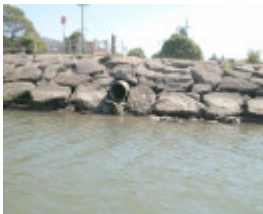
Henderson's Piggery And Wharf Maribyrnong May 2003 Wooden Drain Exit And Wharf Piling
