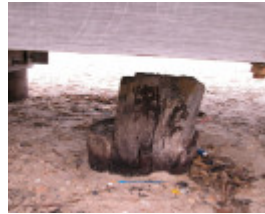
Lagoon Training Walls Wharves And Drain Port Melbourne April 2003 Lagoon Pier Pile 002
