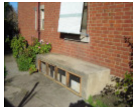
h02087 kahlands winery bendigo air vent 01 aug2005 mz
