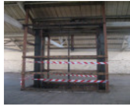
61-9 A'Beckett St lift first floor MZ 24 05 2007
