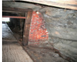
H0198 Wonthaggi State Coal Mine Eastern Precinct H198 July 2007 PM2 air door04
