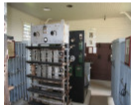
H0198 Wonthaggi State Coal Mine Eastern Precinct H198 July 2007 PM2 lamphouse interior25
