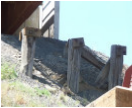
Ingliston Bank railway cutting & piles of remnant railway cutting construction basalt, Moorabool Shire Heritage Study Stage 1, 2010
