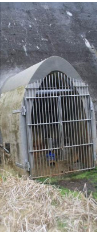
The western valve house.jpg
