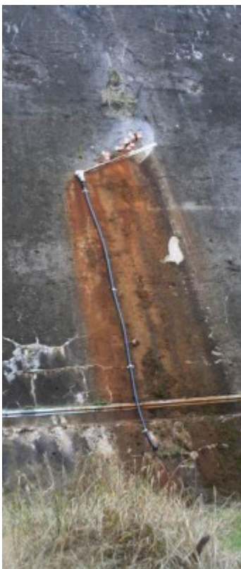
Crack in the dam wall.jpg
