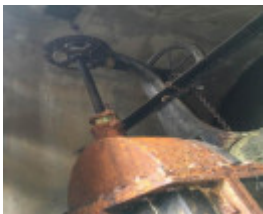
The water supply outlet valve in the eastern house(2).jpg
