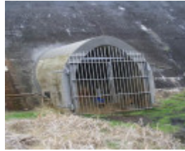
The western valve house.jpg
