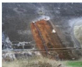
Crack in the dam wall.jpg
