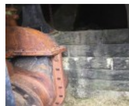
The water supply outlet valve in the eastern house.jpg
