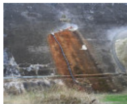
Crack in the dam wall.jpg
