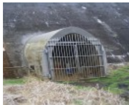
The western valve house.jpg
