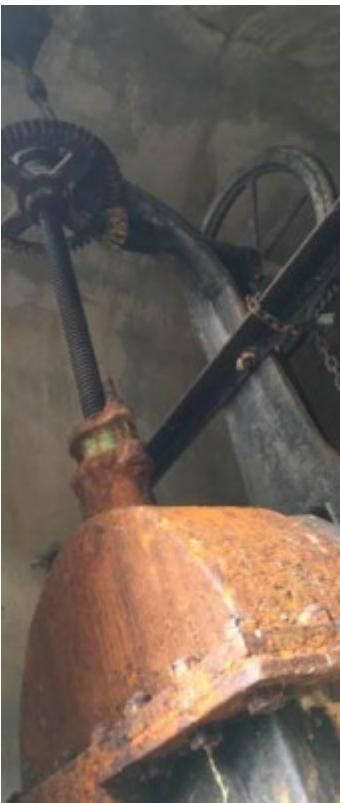
The water supply outlet valve in the eastern house(2).jpg
