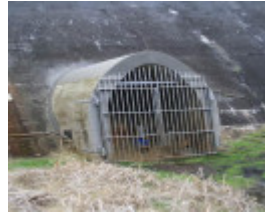
The western valve house.jpg
