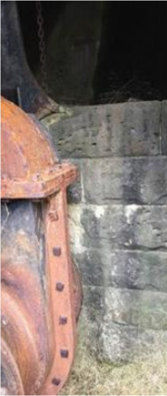
The water supply outlet valve in the eastern house.jpg
