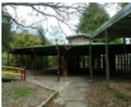
Before Photograph - Reference F3896 2014
