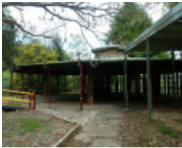
Before Photograph - Reference F3896 2014
