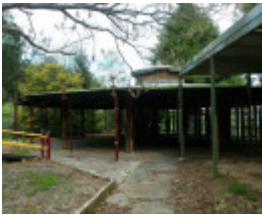
Before Photograph - Reference F3896 2014
