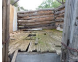
Raised floor and remnant mud and brick pugging to the eastern store
