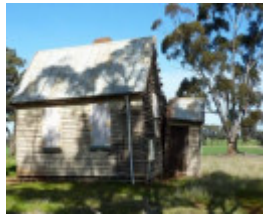
West elevation, note partially detached entrance porch.
