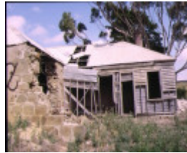
former holy trinity anglican church school merrarp road cees side view mar1993
