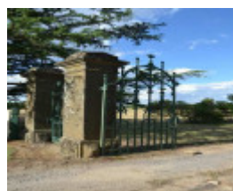
Photo 5 Pillar showing slight damage and rotation.jpg
