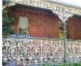
Photo 3: Newtown Brae, detail of east elevation showing delineation in the brickwork (centre) of the original dwelling (right) and single storey front addition (left), February 2016.
