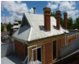
East elevation (first floor) of Building 5, possibly an office or administration building
