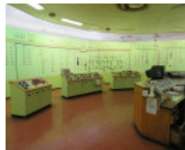
View inside the Power Station Control Room.
