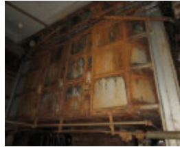
Brown coal fired boiler inside the Power Station.
