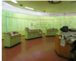
View inside the Power Station Control Room.
