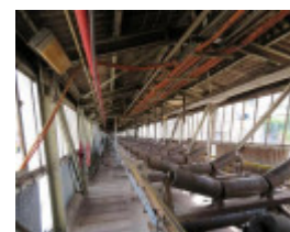
View of the conveyor from North West Corner Station to No.1 Briquette Factory.
