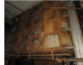
Brown coal fired boiler inside the Power Station.
