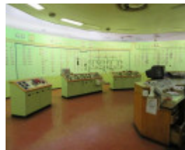
View inside the Power Station Control Room.
