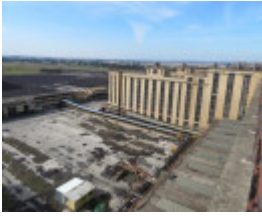
View northeast from the top of No.1 Briquette Factory looking at side of the Briquette Factory (right) and the collecting and feeding conveyors (left)
