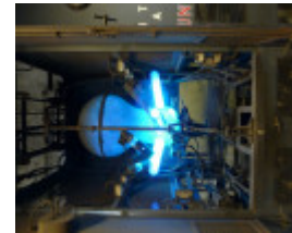
Mercury arc rectifier operating as a number 55 tram approached
