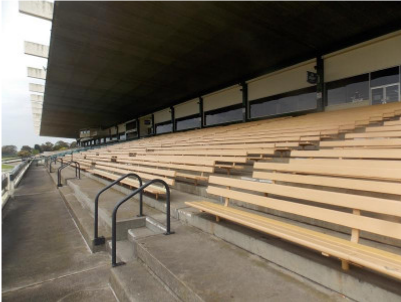
Detail of seating area, showing stepped concrete tier, bench seats and canopy underside.jpg
