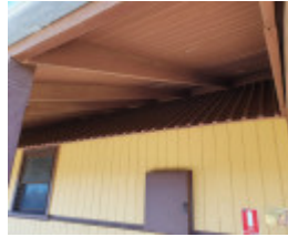
2022, Type A ventilated roof on the Former Irymple Railway Station building showing the battened timber inner roof and ventilator
