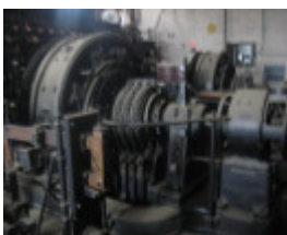
Substation - Rotary converters
