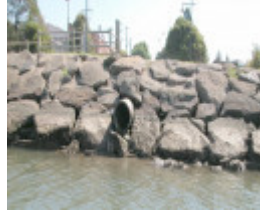
Port Phillip Mills Wharf Maribyrnong May 2003 Wooden Drain Exit And Wharf Piling
