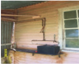
23526 Hillview Nareen electrical system 1982
