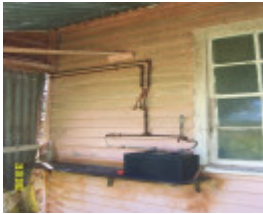
23526 Hillview Nareen electrical system 1982
