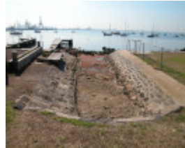
Williamstown Rowing Club Williamstown March 2003 Drain Outlet 002
