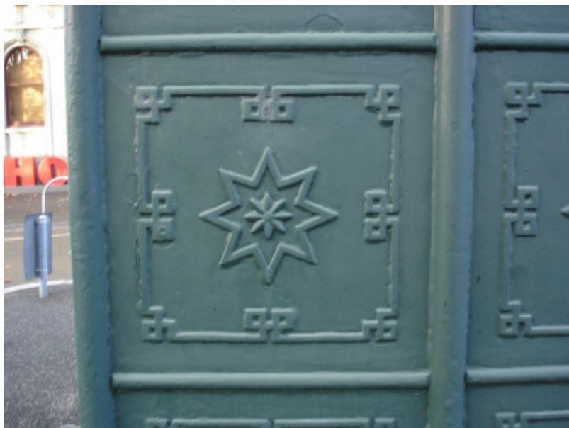
Urinal Nth Melbourne panel detail KJ 21 07 2007
